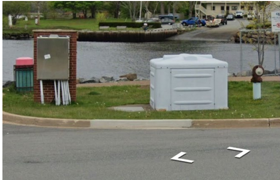
Town Bridge Lift Station
