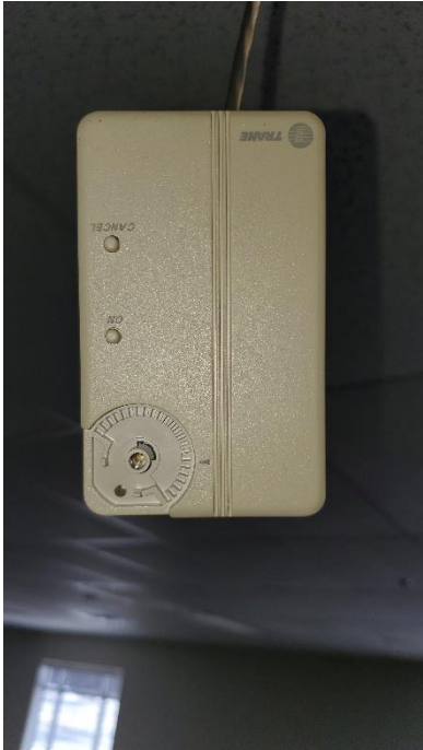
Photo A6: Typical DDC sensor
