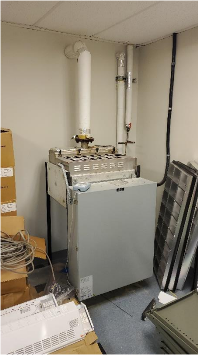
Photo A4: Electric Steam Humidifier
