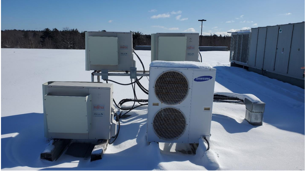
Photo A7: Ductless split units for Server Room
