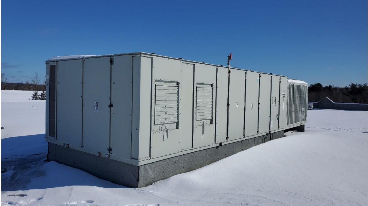
Photo A1: Existing 130 Ton Roof Top Unit
