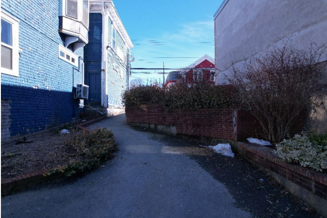
Figure 1. Gorham St walkway looking towards Main St with the existing retaining wall showing signs of deterioration.
