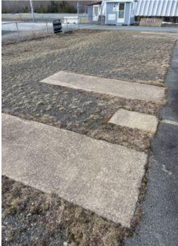
Photo of Aircraft Tie Downs from the airside.
