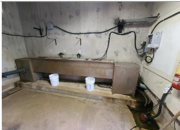
UV Disinfection System
