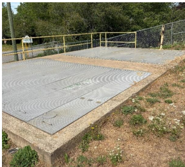
Influent Equalization Tank
