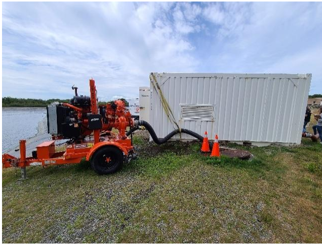
Temporary UV System
