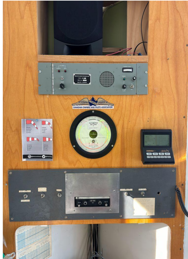
Photo of Altimeter inside the Terminal Building.
