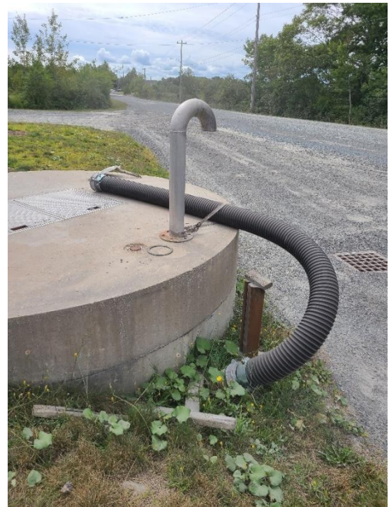
Leachate Discharge Connection at SRS
