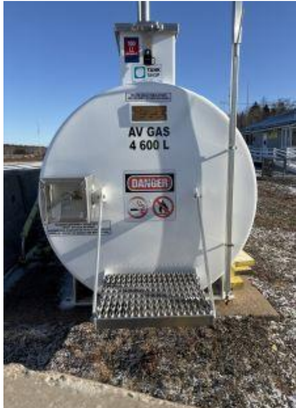
Photo of Avgas Storage and Dispensing from the airside.
