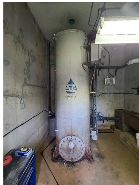
Filtration Unit (Not in Use)
