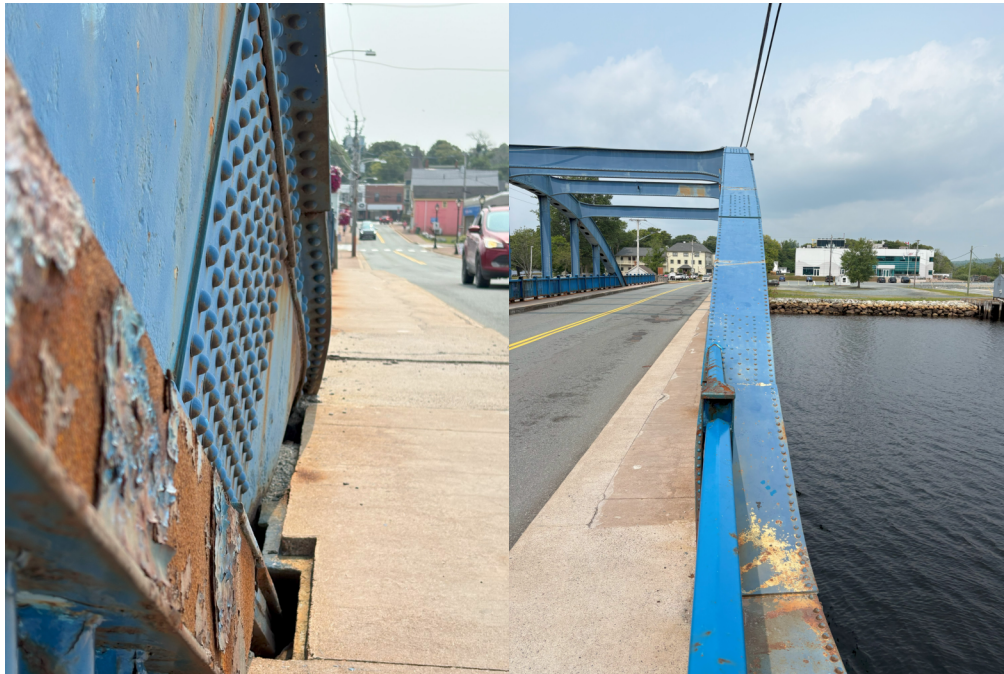
Figure 3 - Buckling observed in the north primary compression member at the east end
